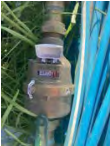
Image 1: Mains Water Supply Meter
