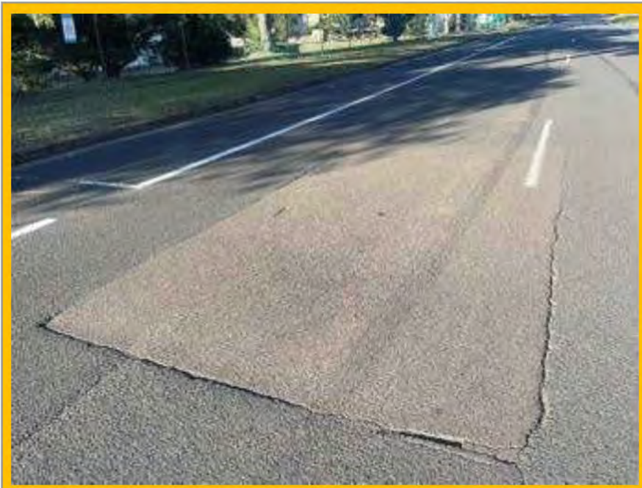
No. 047: cracking at repair to road surface from 261m to 265m
