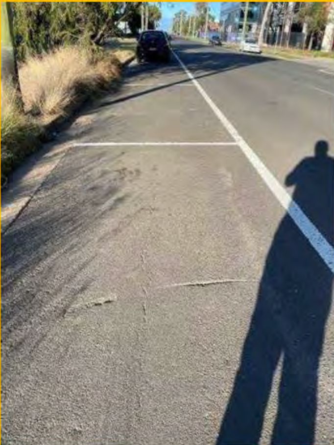
No. 011: Gouge marks on the road surface at approx. 45m
