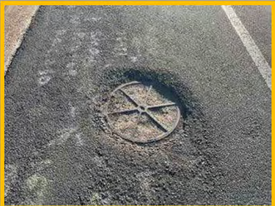
No. 100: depression at manhole cover at 395m
