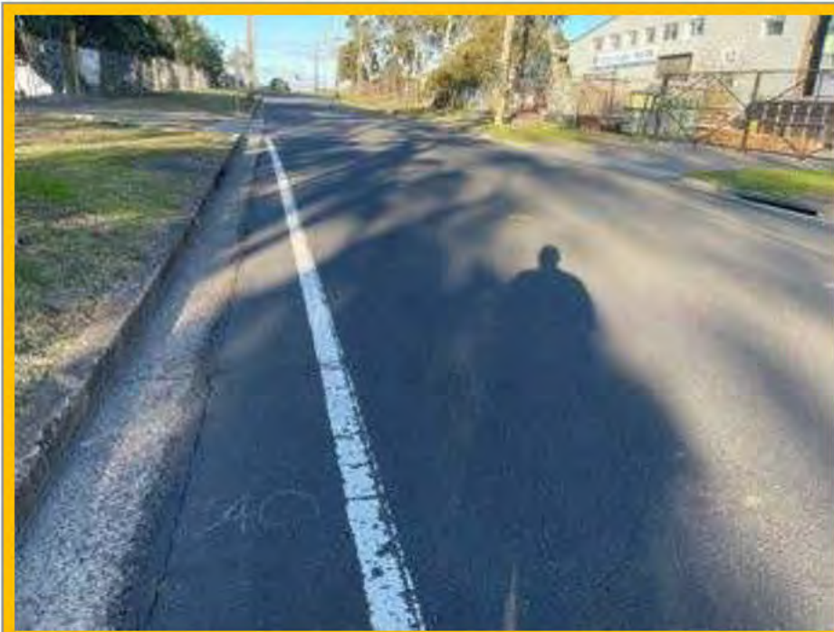
No. 063: 340m. lateral cracking at approx. 341m
