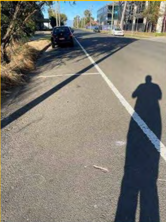
No. 012: 50m. Gouge marks to road surface
