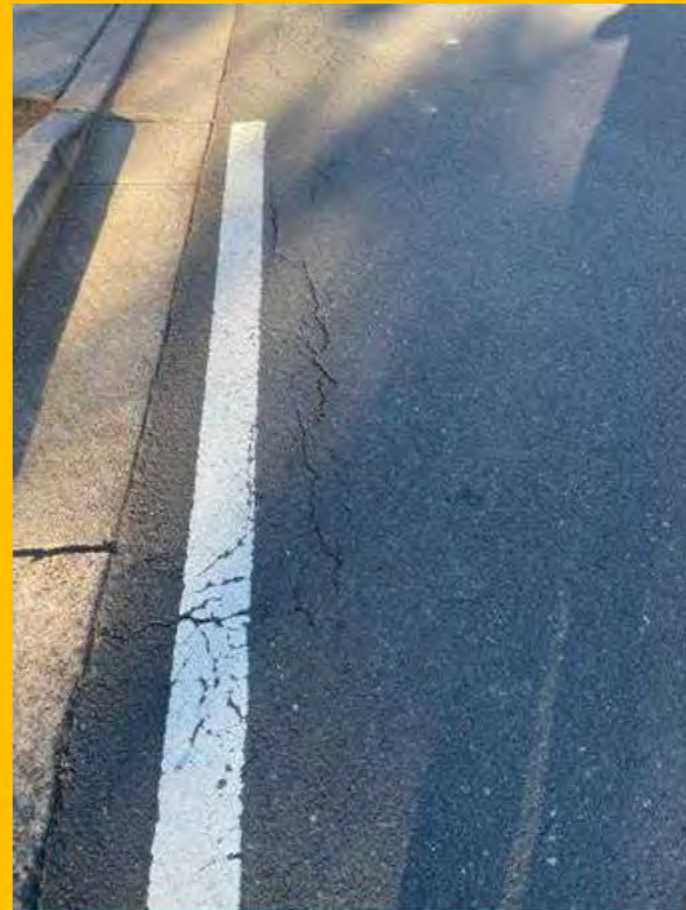
No. 066: continuation of cracking leading to driveway
