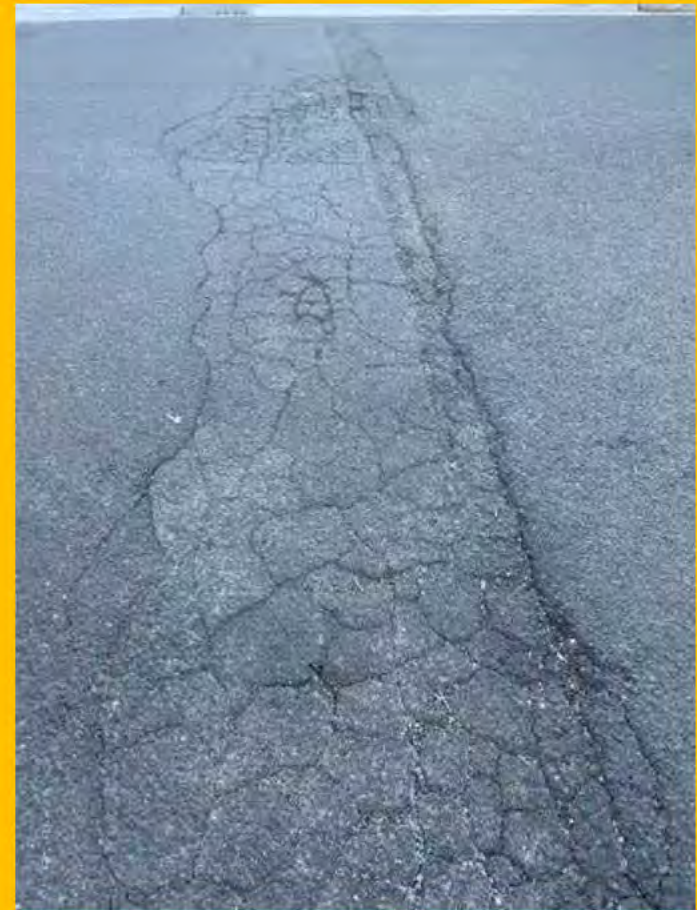
No. 004: deterioration and cracking of previous repairs to road surface
