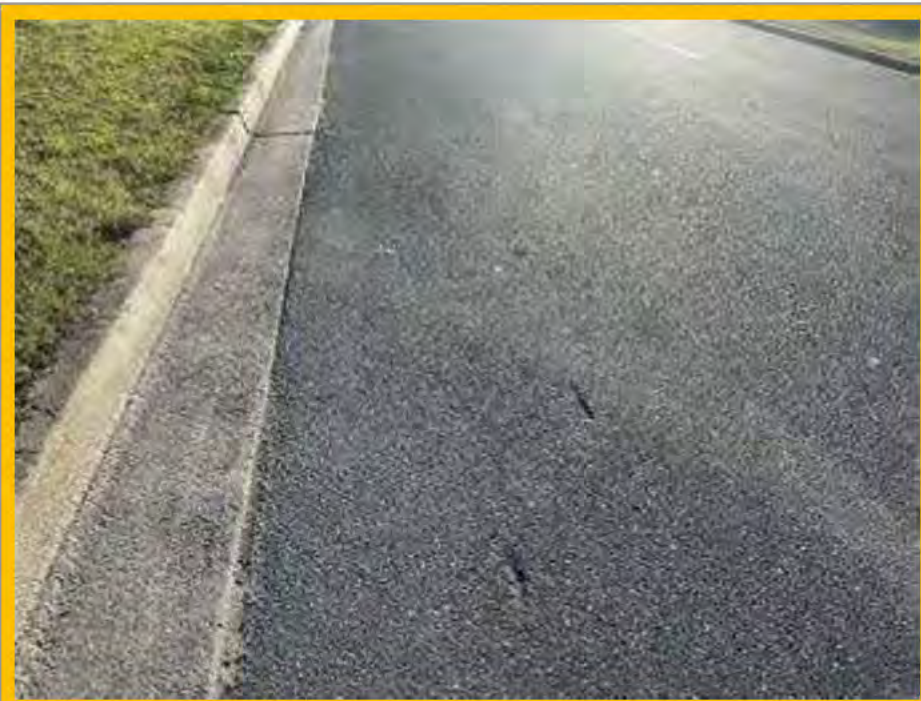
No. 008: gouge marks at 44m
