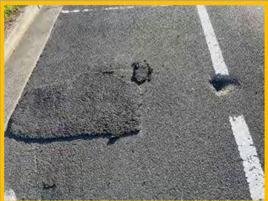
No. 048: road surface repairs and pothole at approx. 229m
