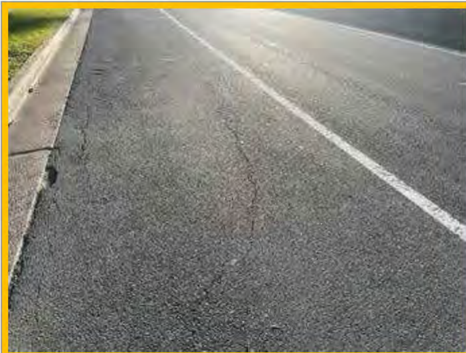
No. 075: damage at kerb line at 299m and cracking in parking bay road surface from 299m to 302m
