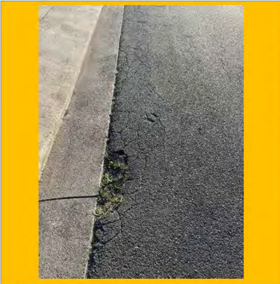
No. 089: damage to kerb line at layback to western end of 24 Harris St
