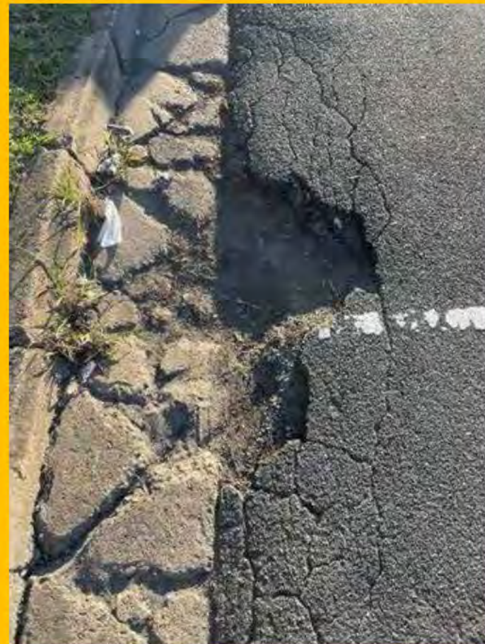
No. 124: damage to road surface and kerb line at 512m
