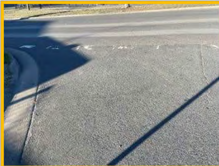
No. 091: longitudinal cracking commencing approx. 3m from intersection at Glossop St
