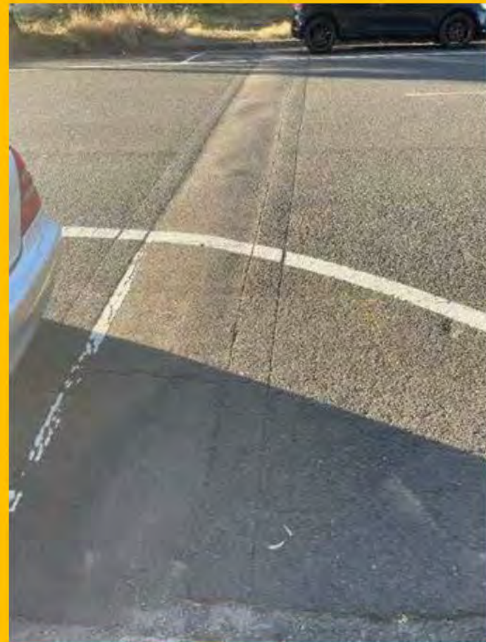
No. 120: cracking and repairs to road surface extending across full width of road at 491 m
