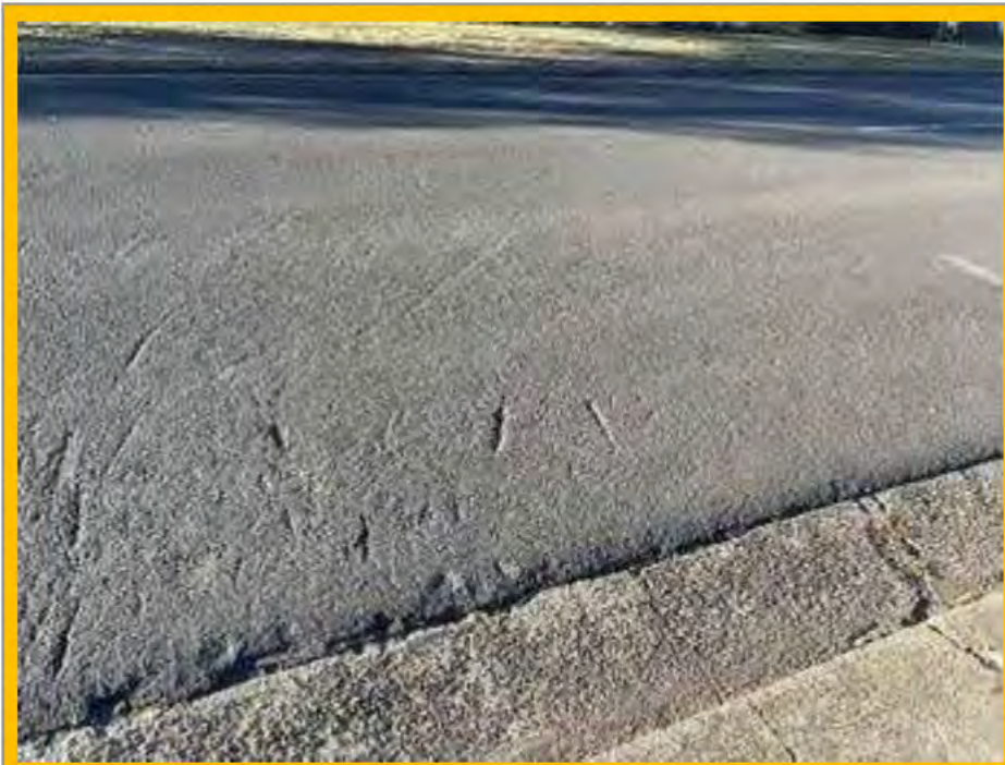
No. 031: gouge marks at 8 Harris St
