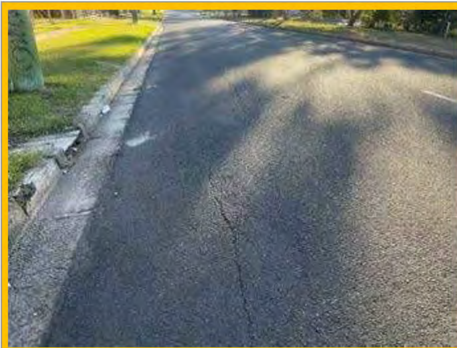
No. 025: continuation of cracking from 110-120m
