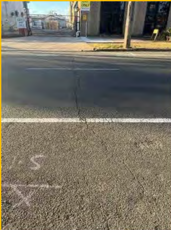
No. 111: lateral crack extends across full width of road
