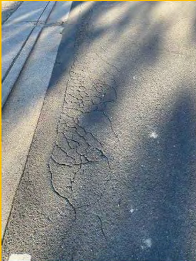
No. 067: damage to road surface at layback to 17 Harris St (356m to 364m)
