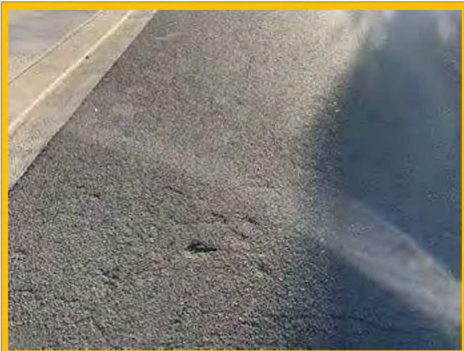
No. 117: gouging to road surface at 476m
