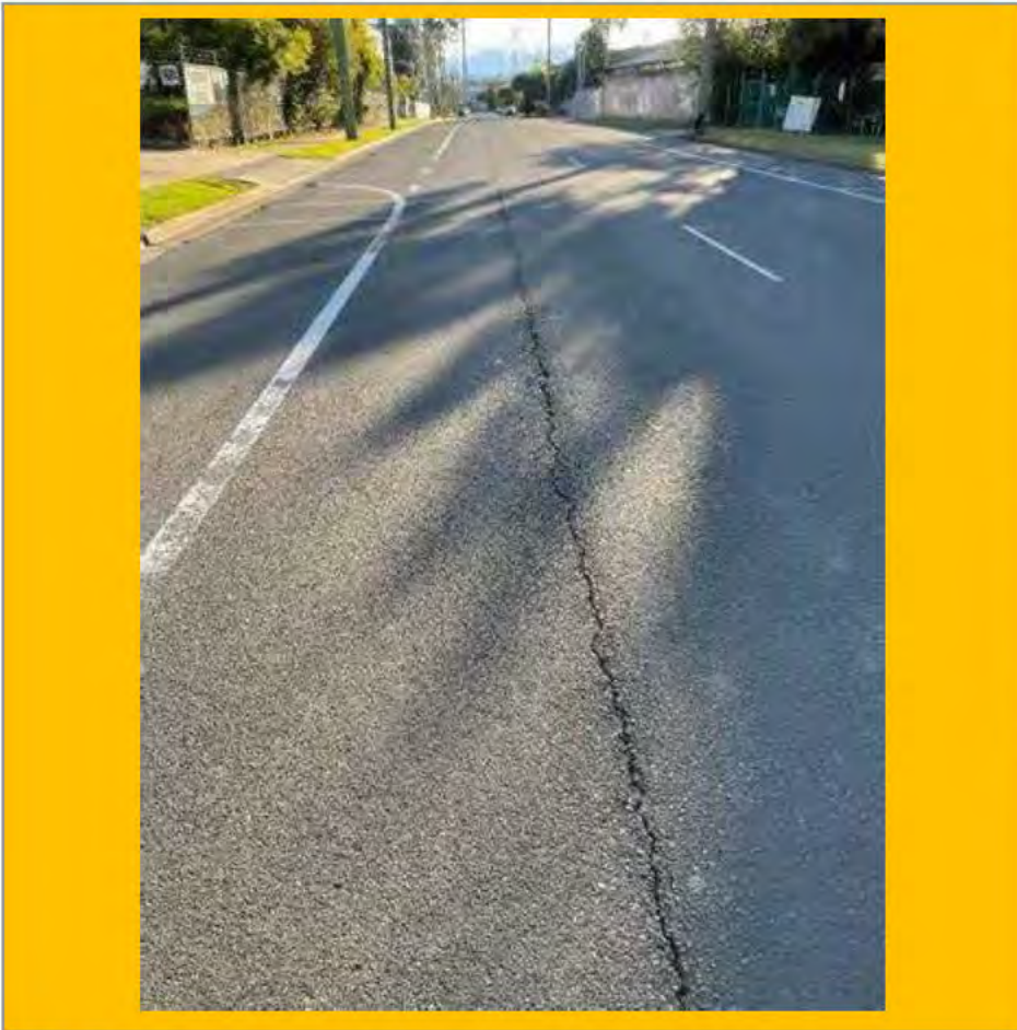
No. 055: continuation of crack in road centre
