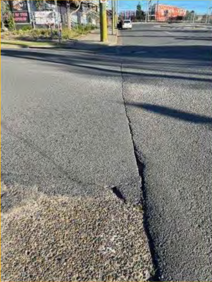
No. 002: Western end of Harris Street as it abuts Forrester Road. There is a crack at the join in road surfaces at this intersection and minor damage present.
