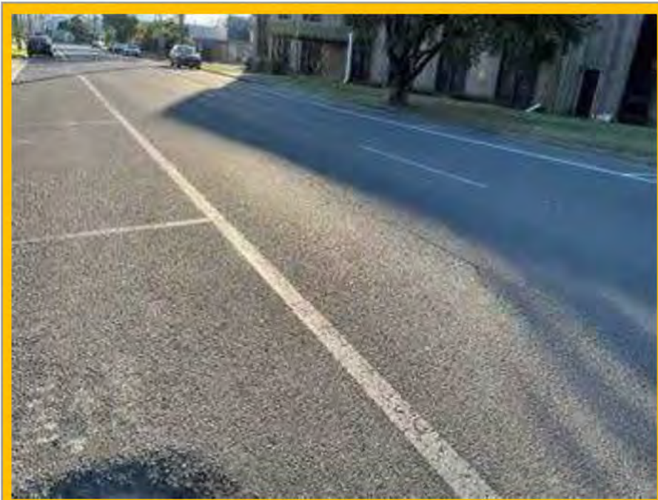
No. 101: crack in road join materials
