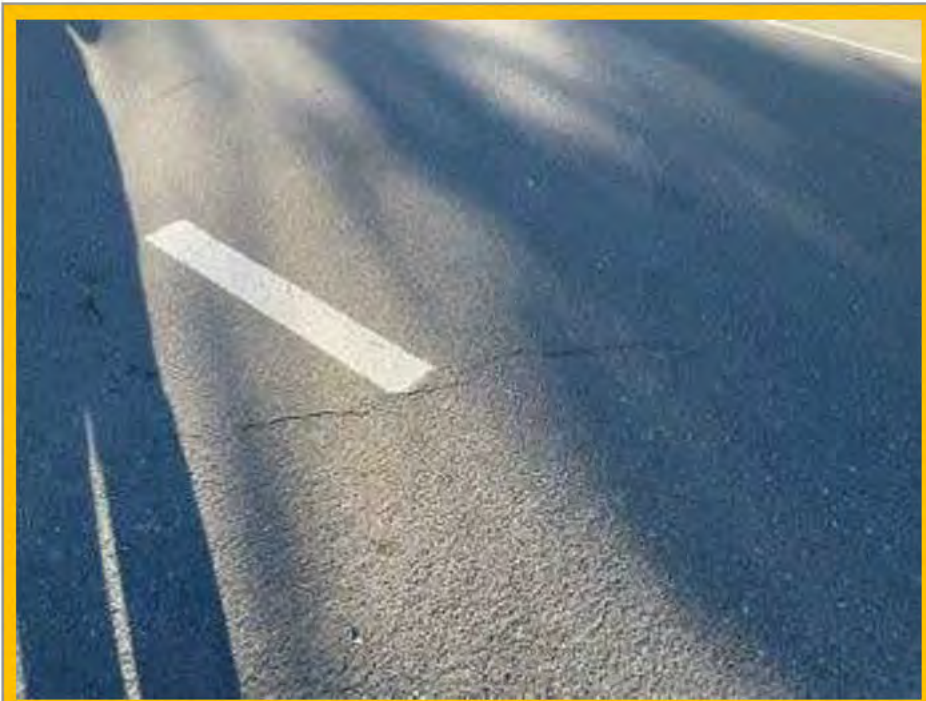
No. 059: lateral cracking at 31.5m
