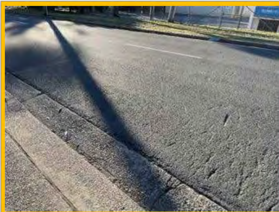
No. 033: gouge marks at 8 Harris St
