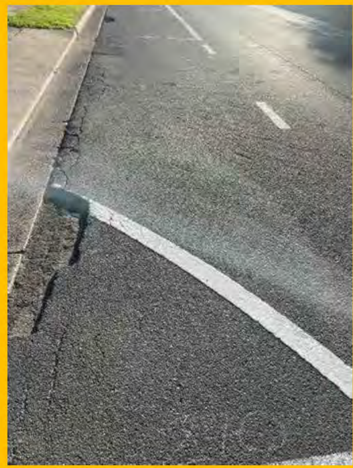
No. 062: damage to road surface at eastern layback to 24 Harris St
