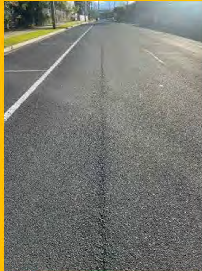
No. 068: continuation of crack in road centre
