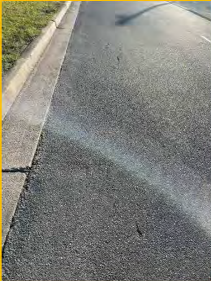
No. 009: gouge marks at 45-50m
