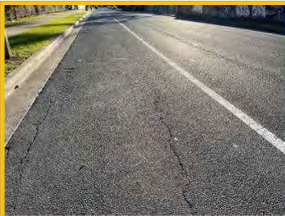
No. 076: 300m. continuation of cracking in road surface in parking bay
