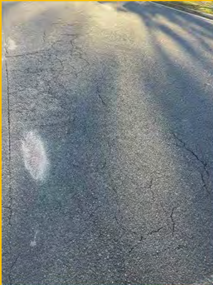
No. 041: deterioration and cracking to road surface from 190 to 193m at layback to 14 Harris St
