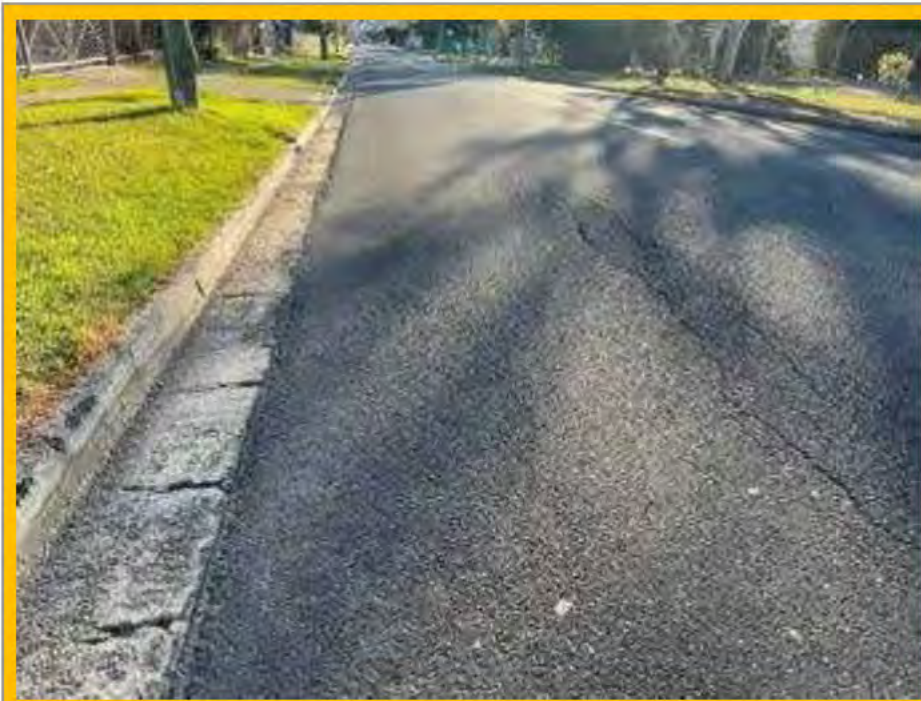
No. 027: 130m. indentation to road surface and cracking continues
