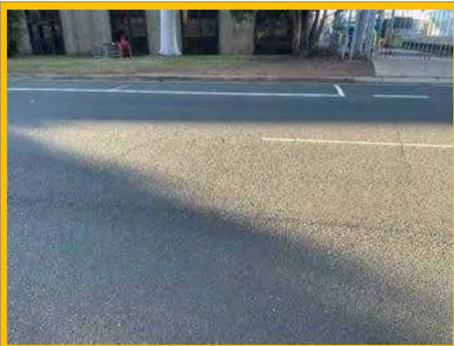
No. 097: lateral cracking to road centreline at 375m
