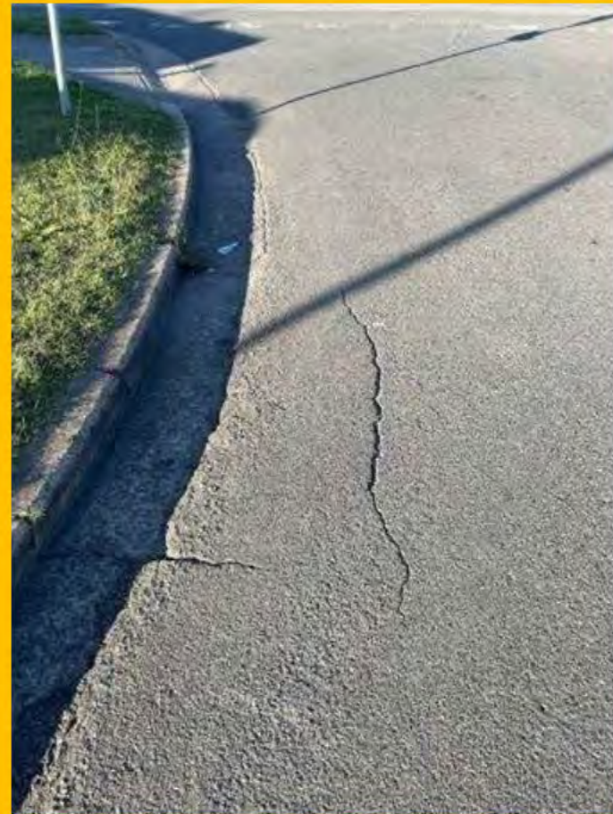
No. 090: Cracking and damage to kerb line at corner at approx. 545m
