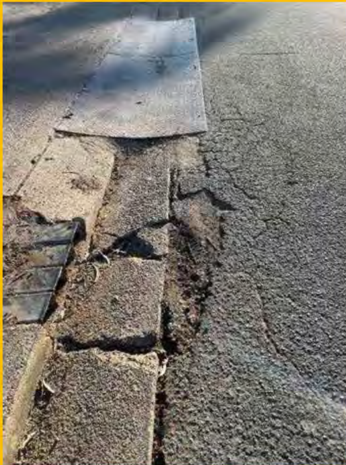
No. 021: damage at 6 Harris St
