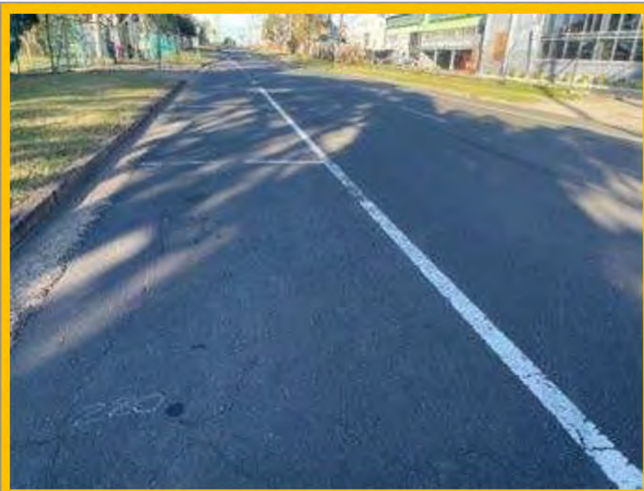
No. 051: 280m. Cracking in surface from approx. 279m to 283m
