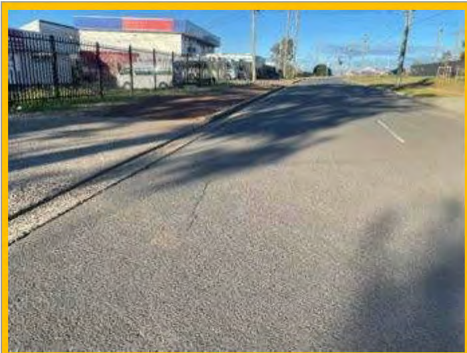
No. 077: cracking parallel to layback at 7 Harris St
