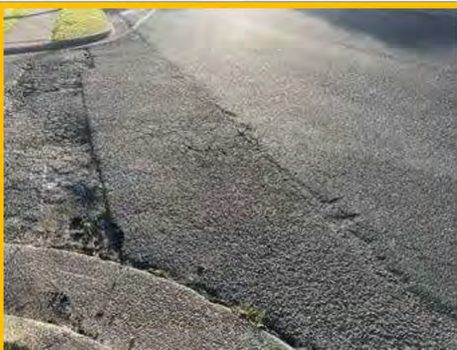
No. 095: deterioration of road surface repairs
