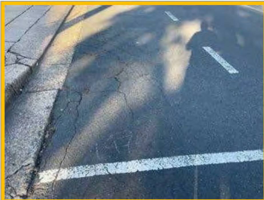
No. 037: damage radiating out from the layback at entrance to 21 Harris St (197m)
