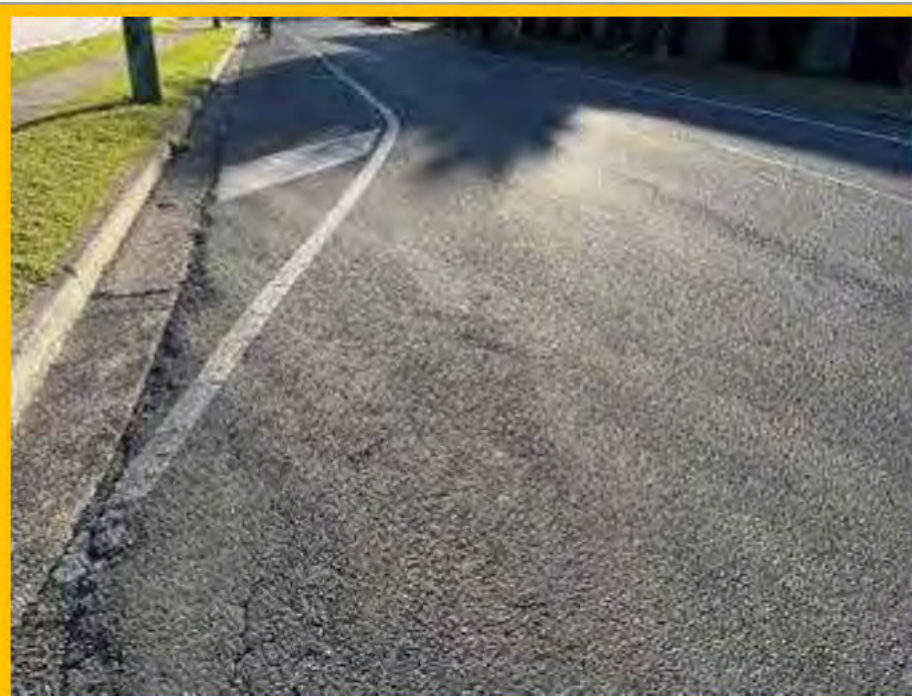
No. 096: 370m. deterioration to road surface radiating west from car park entrance
