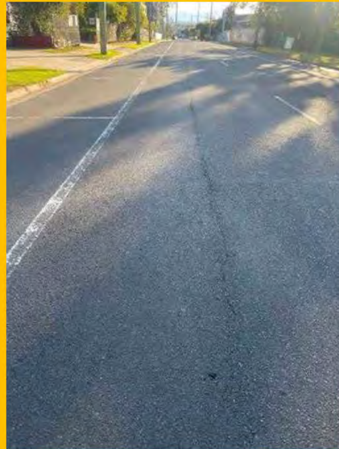
No. 052: longitudinal crack in road centre at joint in materials commences from approx. 240m and continues through to approx. 290m
