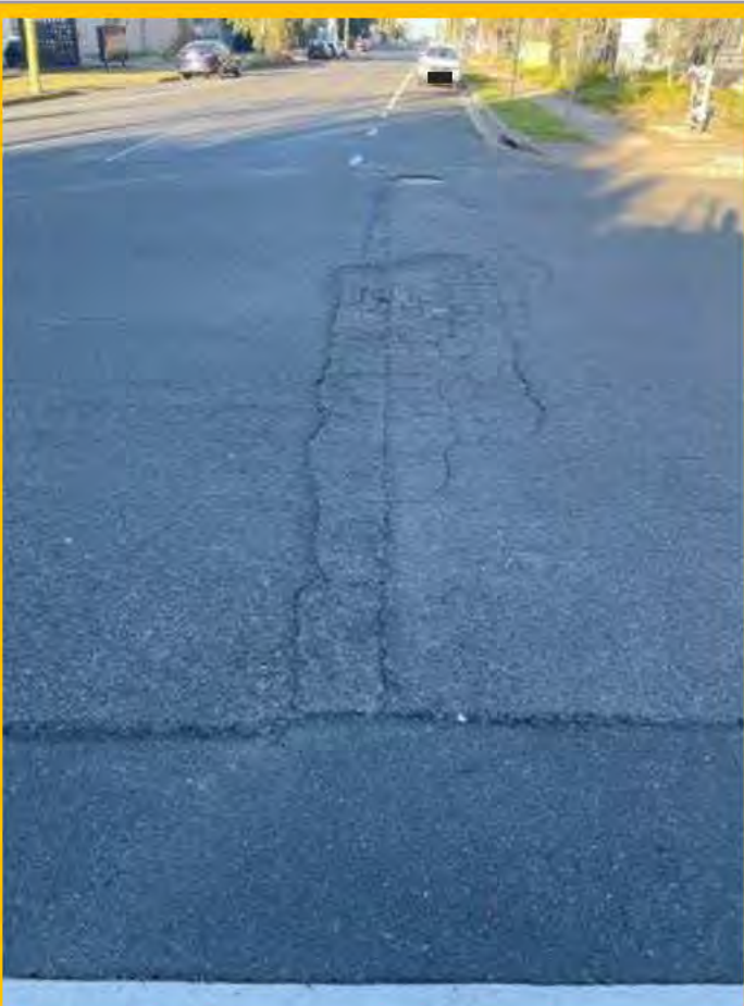
No. 002: Deterioration to road surface from intersection to Harris Street across full width of Forrester Road, viewed from ACFS/Pacific National facility entrance (2 Forrester Rd)
