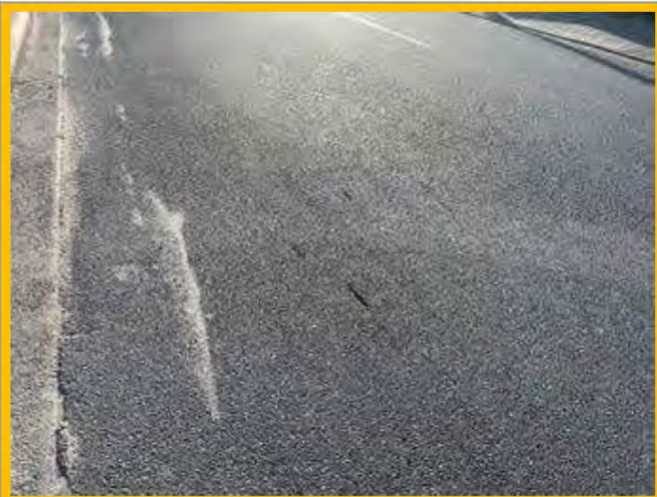
No. 006: general deterioration at 30m and beyond, and gouge marks at approx. 35m
