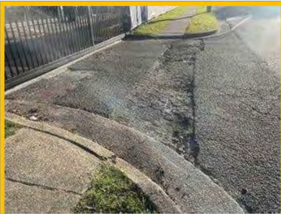
No. 094: significant damage to car park entrance
