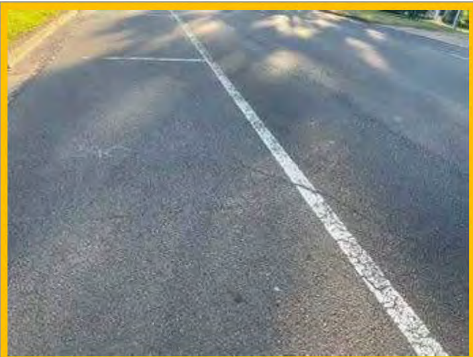
No. 050: cracking to road surface at 239m
