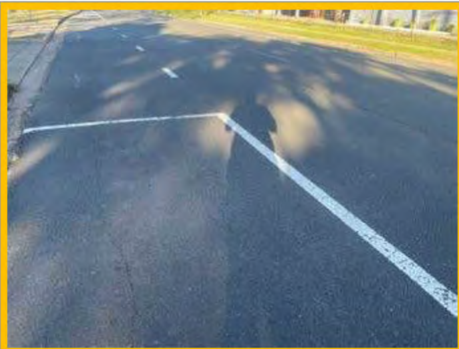
No. 054: longitudinal cracking from 293m to 300m
