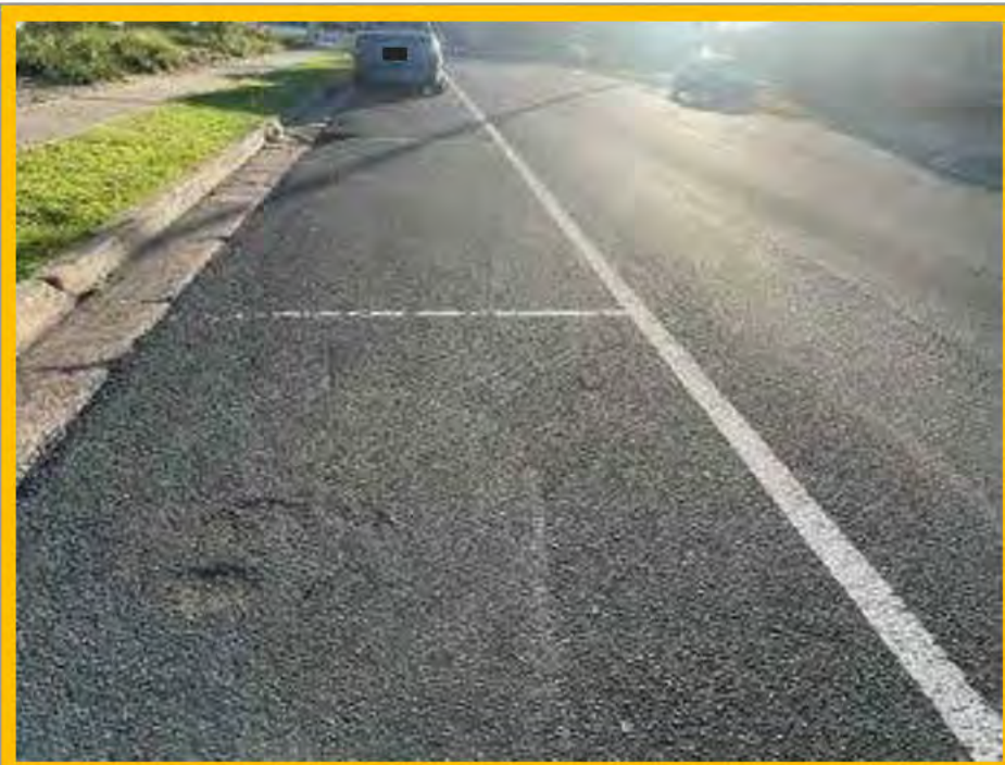
No. 122: indentation in parking bay road surface at 503m
