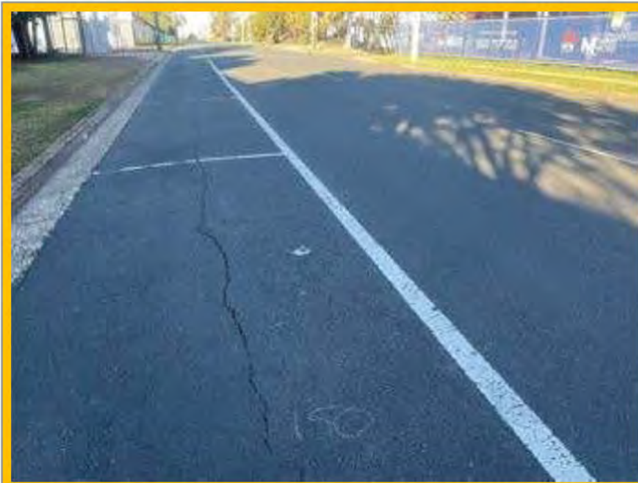
No. 027: Longitudinal cracking in road surface from approx. 150m to 158m
