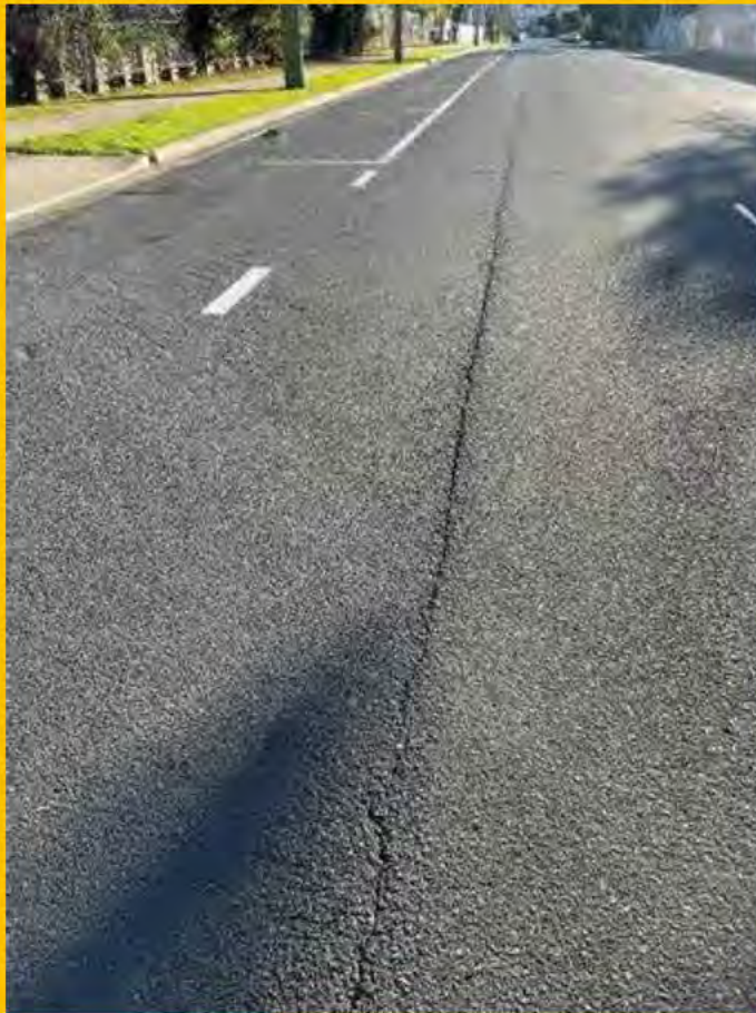
No. 063: continuation of crack in road centre
