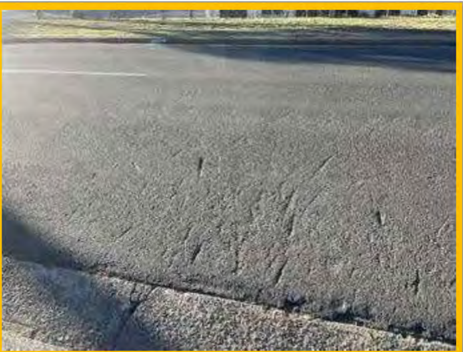
No. 032: gouge marks at 8 Harris St
