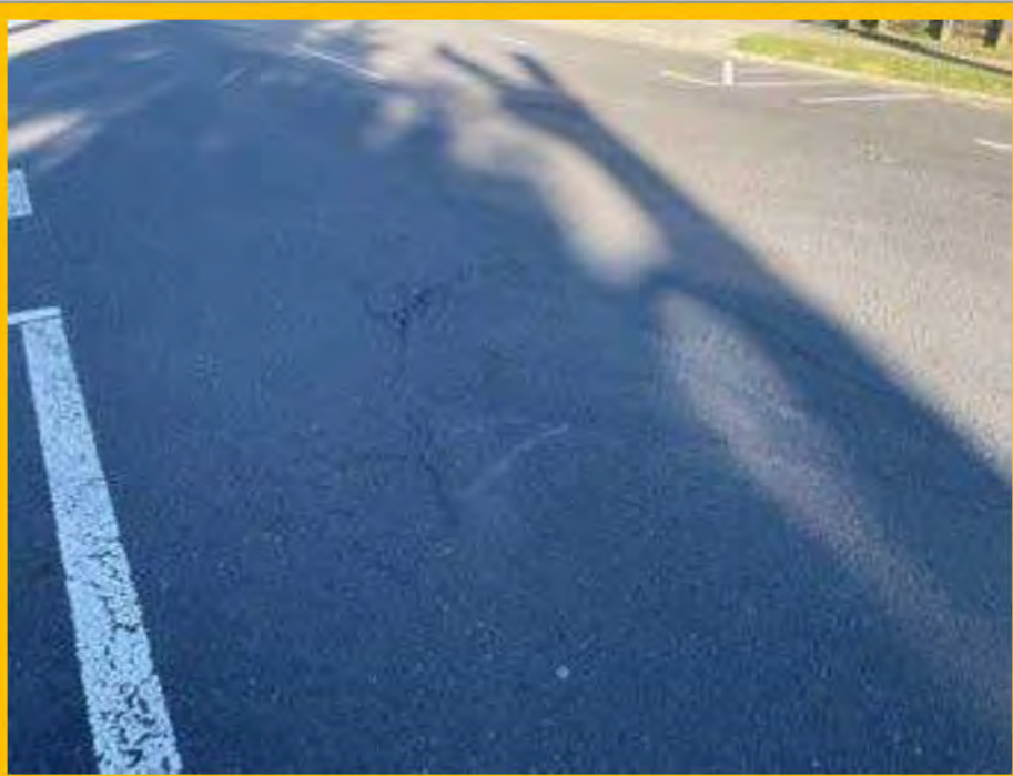
No. 036: cracking in surface at approx. 194, 195m
