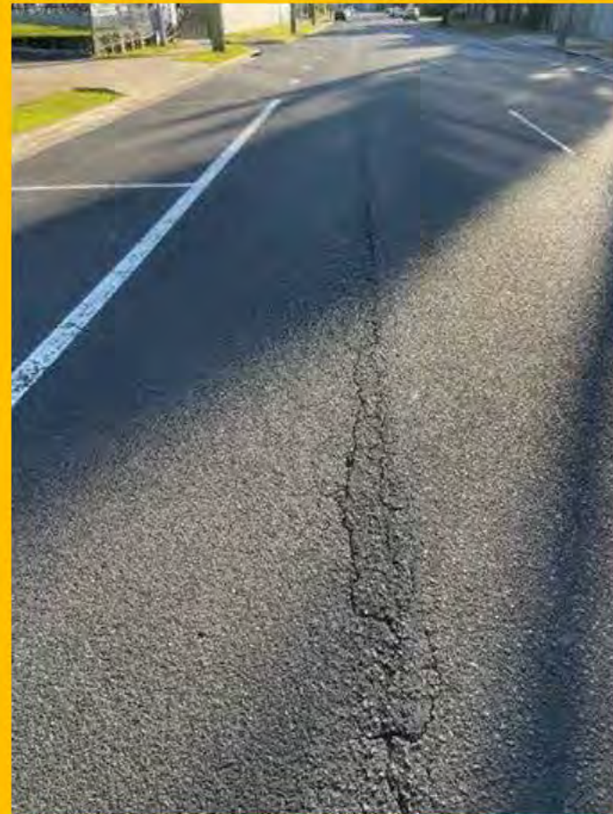
No. 086: continuation of crack in road join materials
