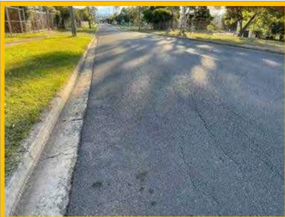
No. 026: 120m. multiple cracks continuing from 120m and beyond
