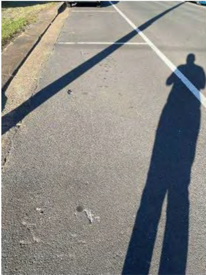
No. 005: Gouge marks on the road surface
