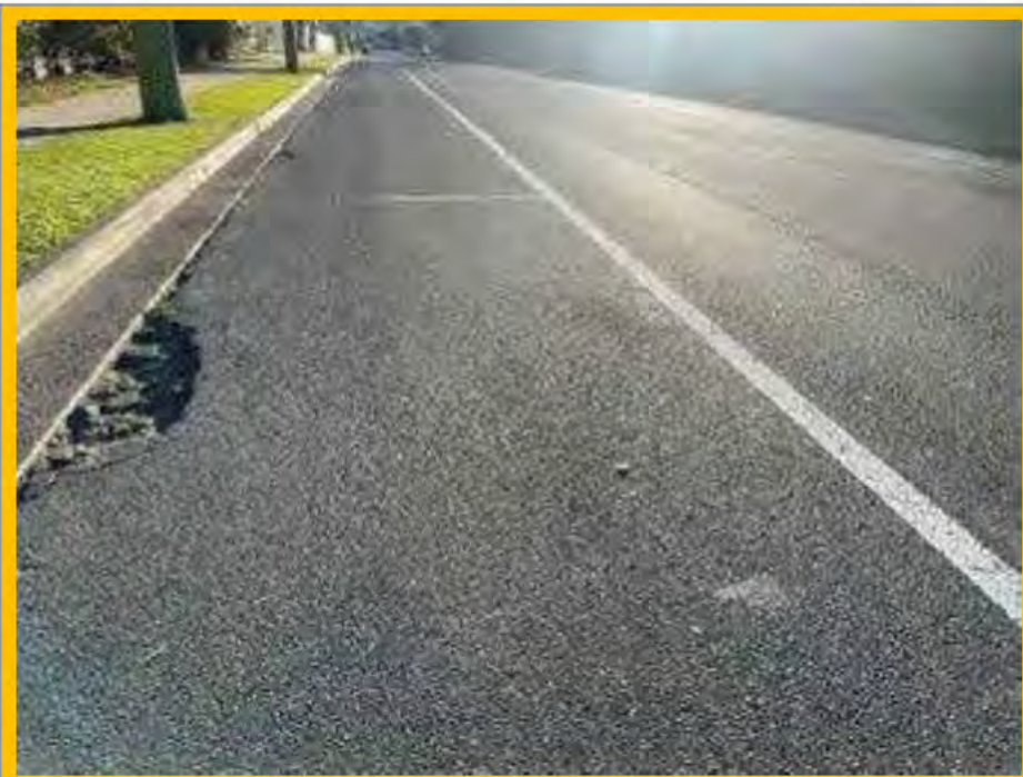
No. 066: 280m. Damage to road surface at kerb line at 281m
