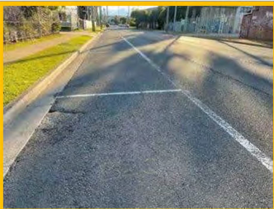
No. 082: 320m. continuation of parking bay surface cracks
