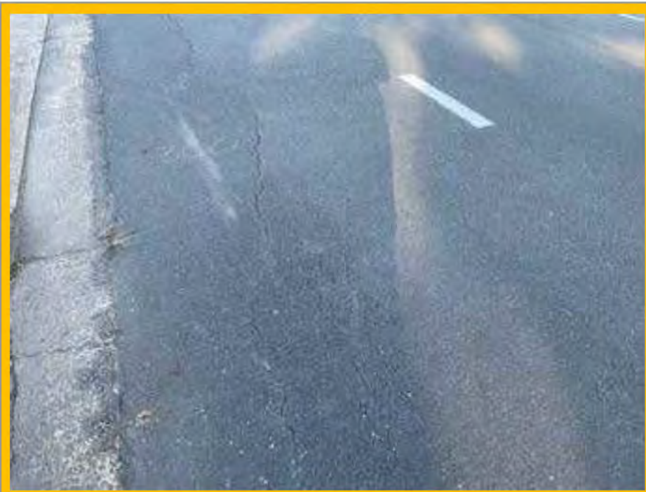
No. 055: longitudinal cracking from 298m to 310m
