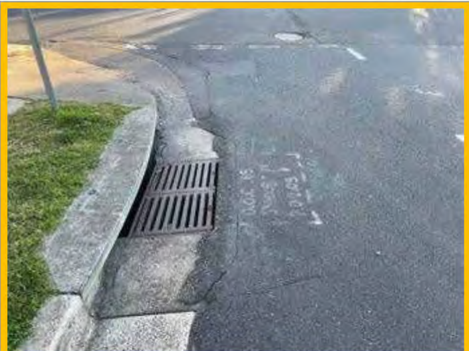
No. 128: cracking to road surface parallel to stormwater drain and at joints in road materials for previous repairs
