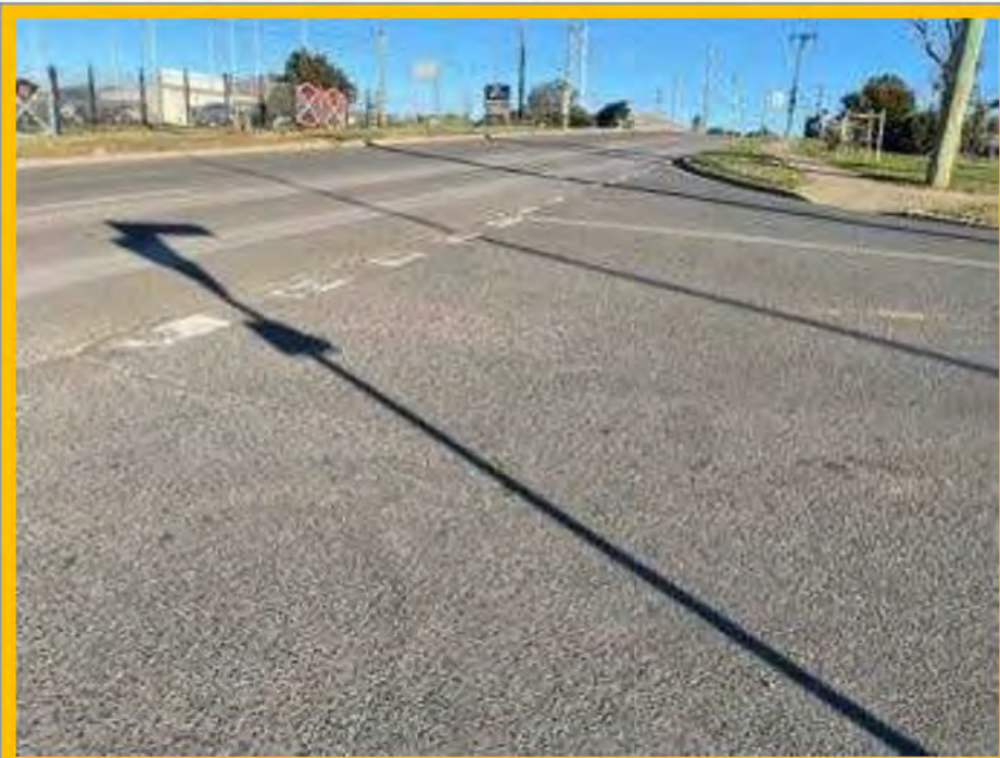
No. 092: Eastern end of Harris Street as it abuts Glossop St. There is a crack at the join in road surfaces at this intersection and minor damage present.
