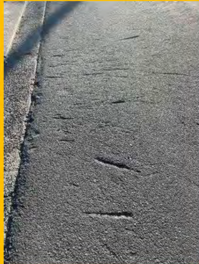
No. 030: gouge marks at 8 Harris St
