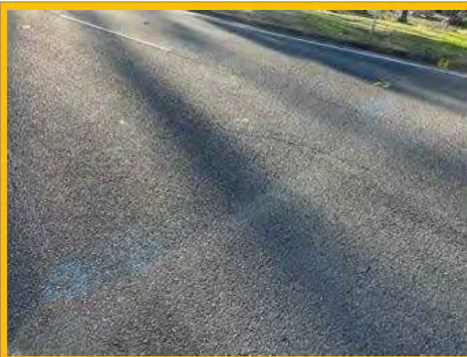
No. 043: longitudinal cracking at road centre at approx. 208m
