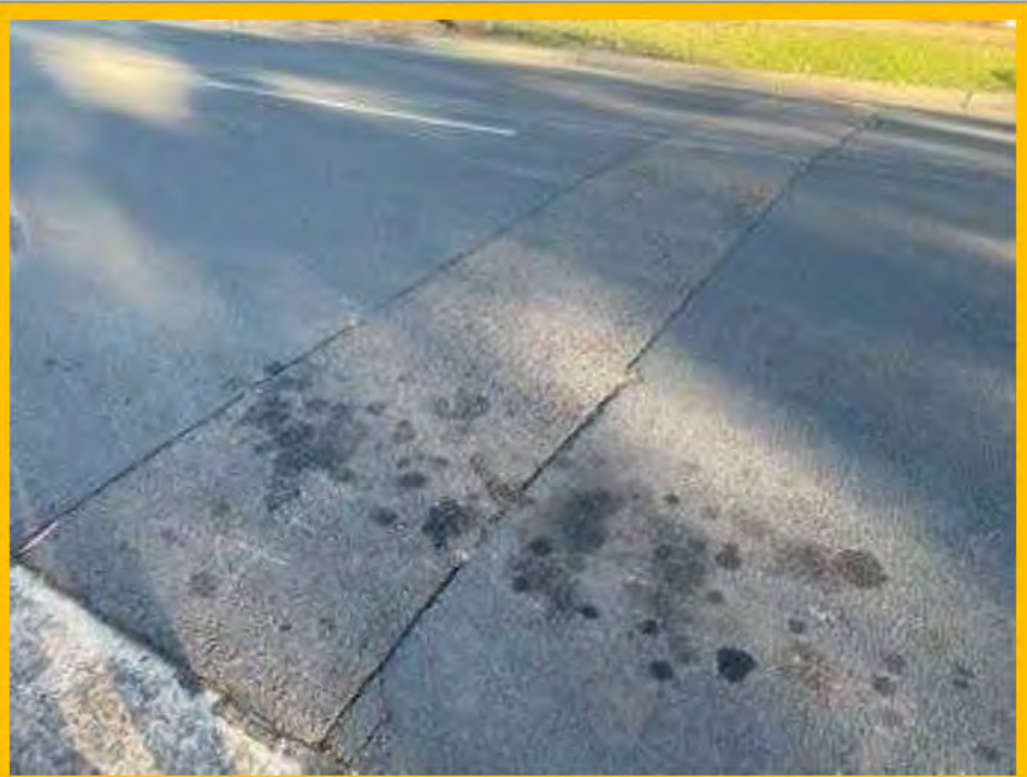
No. 082: Repairs to road surface across width of street at approx. 474m
