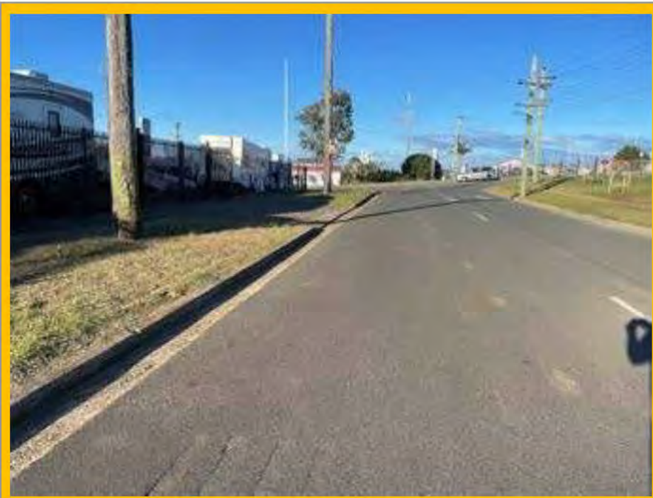
No. 085: 500m. Gouging to road surface at approx. 499m
