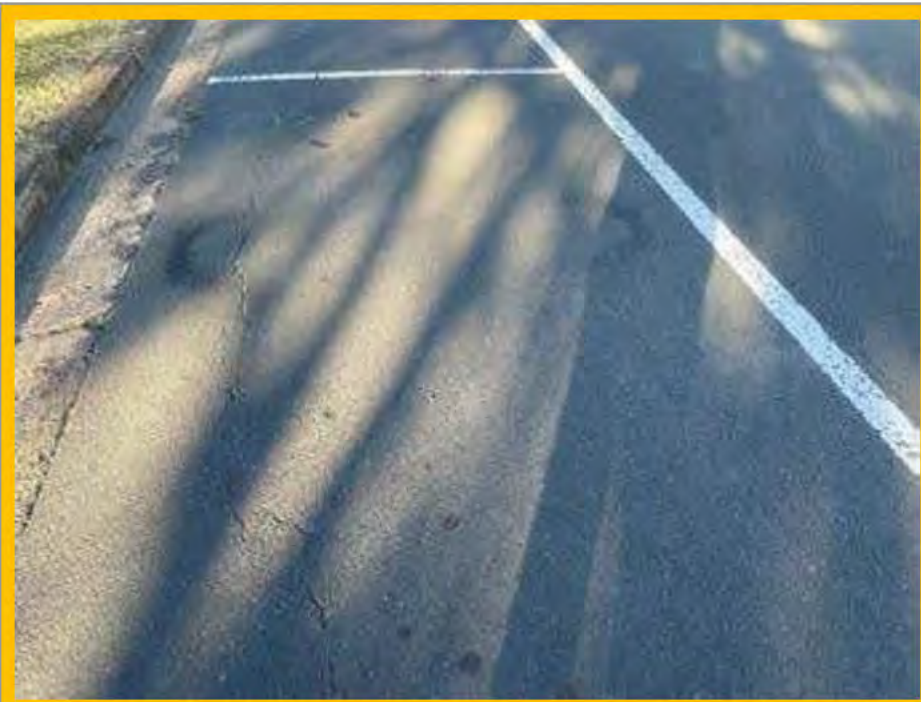
No. 052: longitudinal cracking in surface from approx. 286m to 290m
