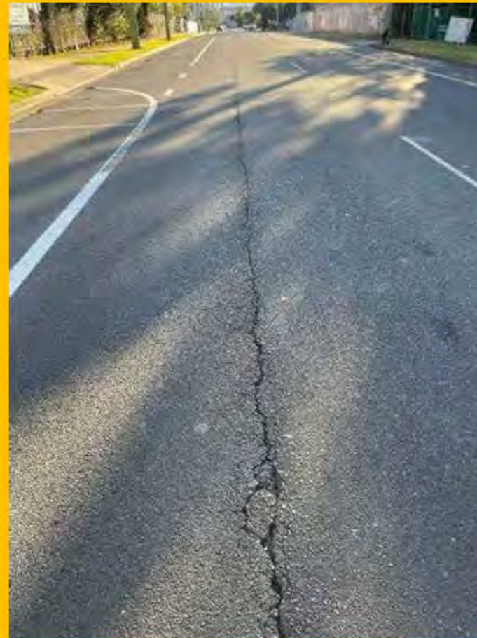
No. 058: continuation of crack in road centre
