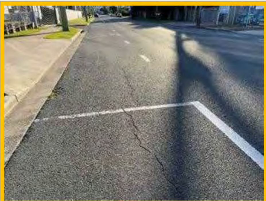
No. 088: 340m. continuation of parking bay surface cracks to 345m
