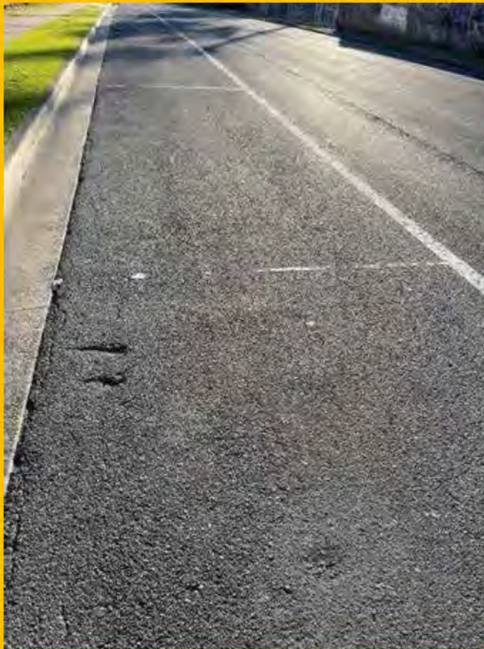
No. 077: gouge marks in road surface at 304m
