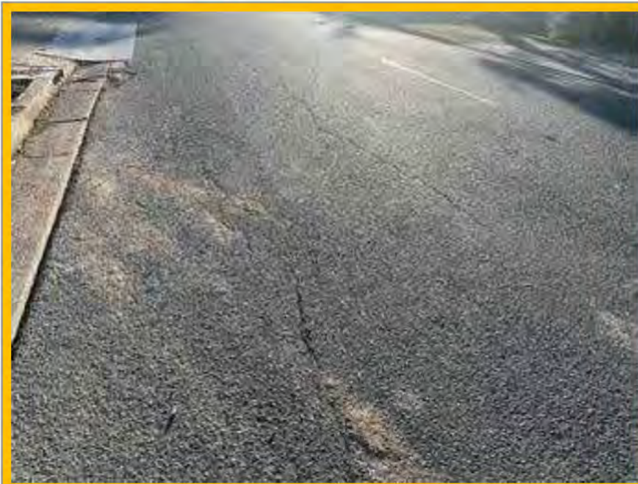
No. 019: multiple longitudinal cracks from approx. 92m and beyond
