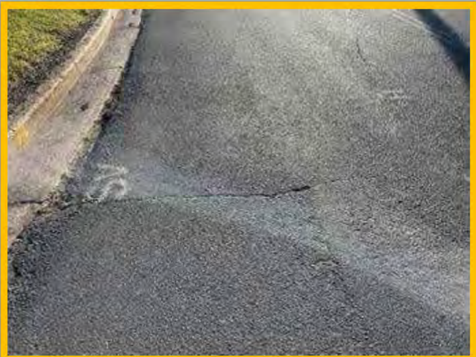
No. 002: varying cracks to the road surface 5m from southeast corner
