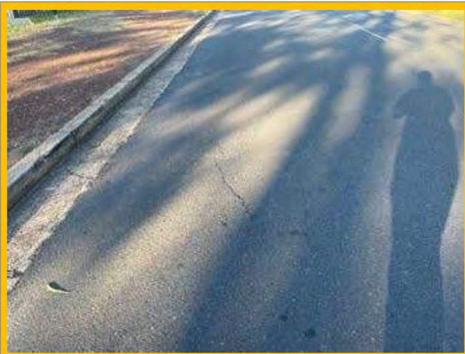
No. 079: cracking in road surface at approx. 456m
