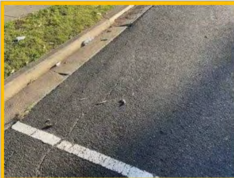
No. 109: various cracks parallel to kerb line from approx. 445m
