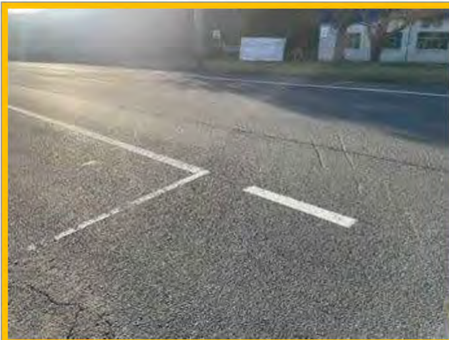
No. 065: gouging toward road centreline at eastern layback to 24 Harris St (approx. 274m)
