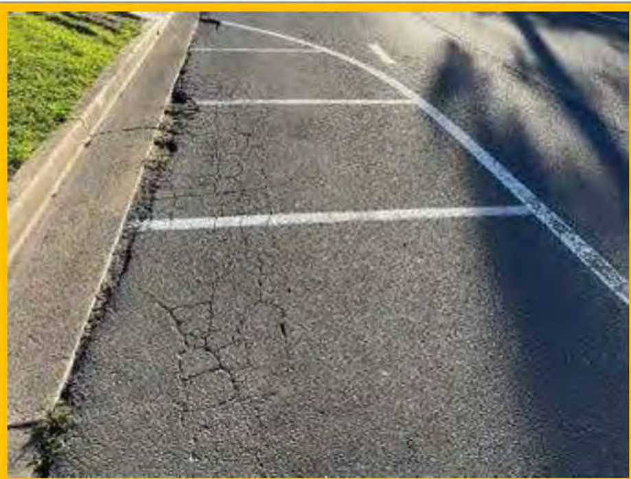
No. 060: deterioration of road surface adjacent to kerb line from 265m to 270m
