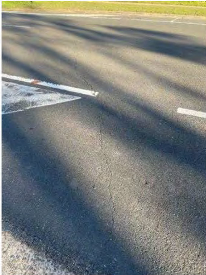
No. 061: lateral cracking from kerbline to centre of road at approx. 323m
