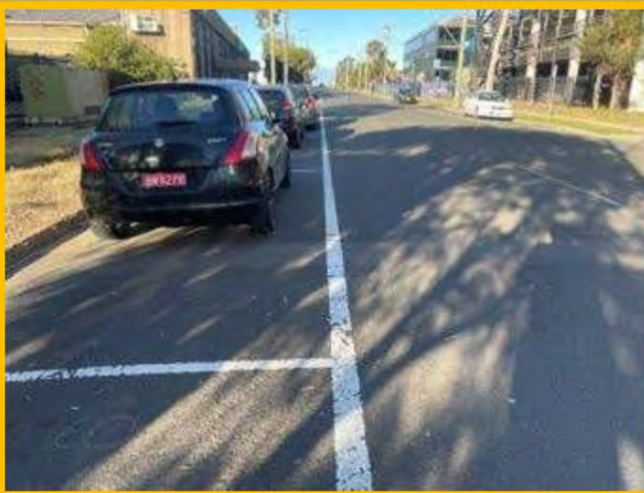
No. 013: 60m. Repairs to road surface across width of street at approx. 62m
