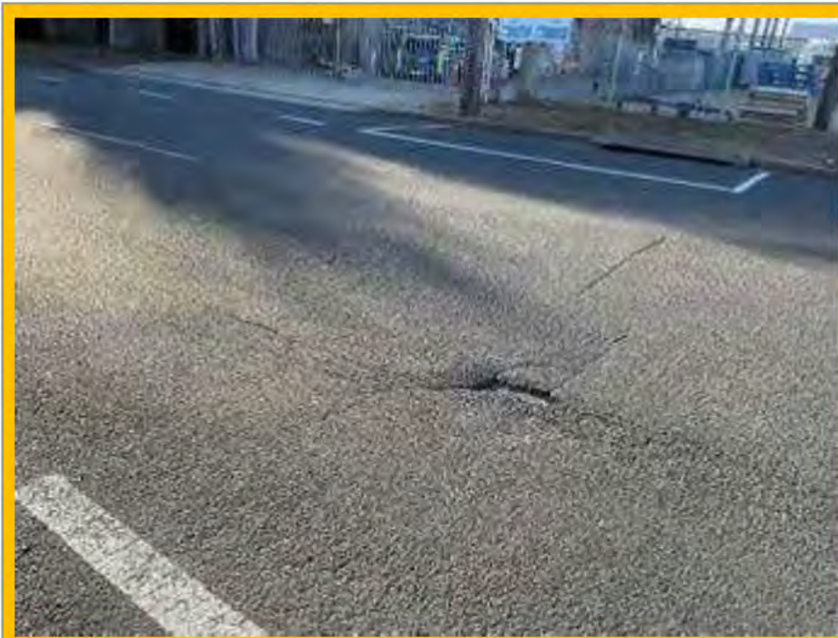
No. 091: damage and surface cracks at 355m
