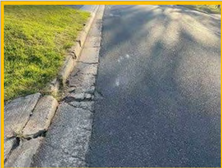
No. 039: damage at layback to 12 Harris St (approx. 183m)
