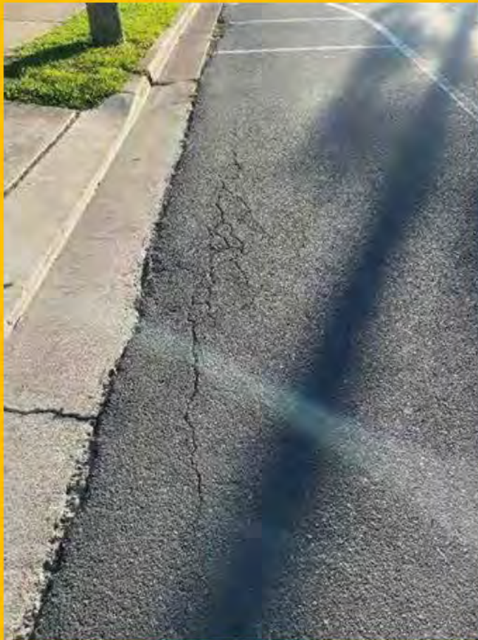
No. 057: cracking and deterioration of road surface at western layback to 14-16 Harris St
