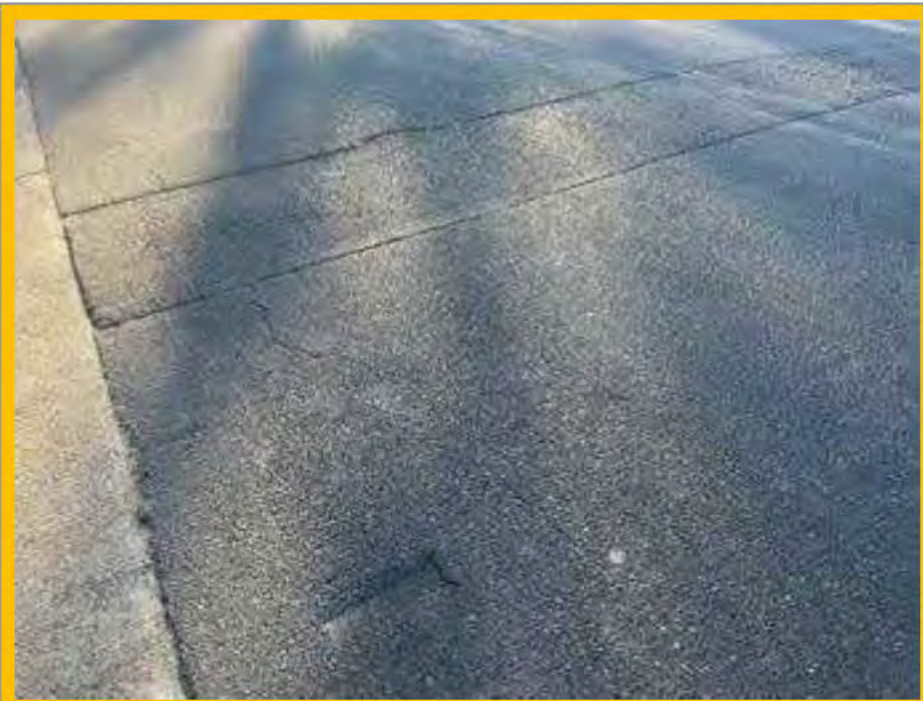
No. 014: repairs to road surface across width of street at approx. 78m
