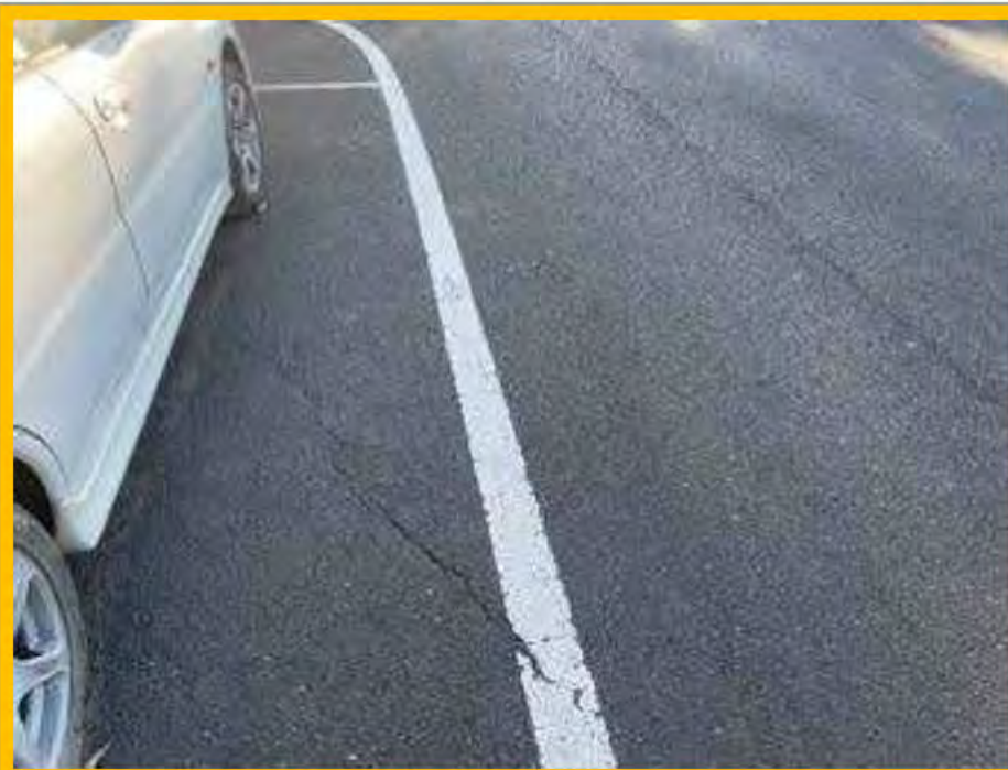
No. 113: continuation of crack in parking bay road surface at approx. 465m
