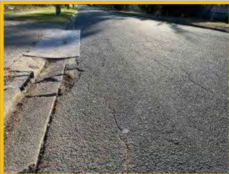
No. 020: 100m. continuation of cracking. Significant damage to road surface and layback at 6 Harris St
