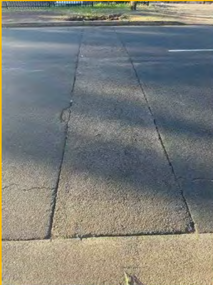
No. 015: repairs to road surface across width of street at approx. 78m
