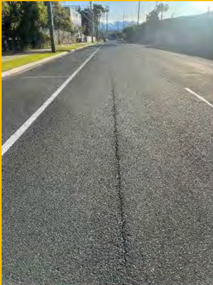
No. 069: continuation of crack in road centre
