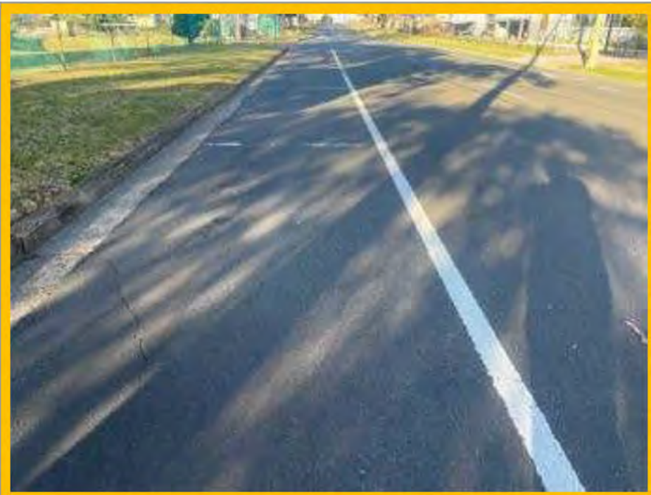
No. 048: cracking in surface at approx. 268m
