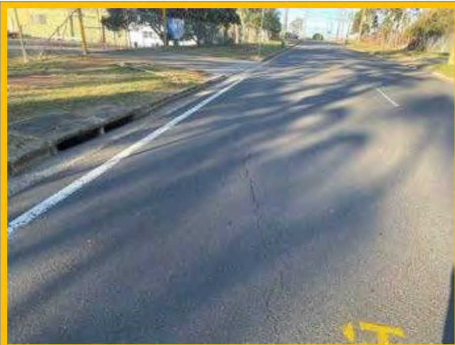
No. 064: cracking from centre of road leading toward kerblines at approx. 344m to 352m
