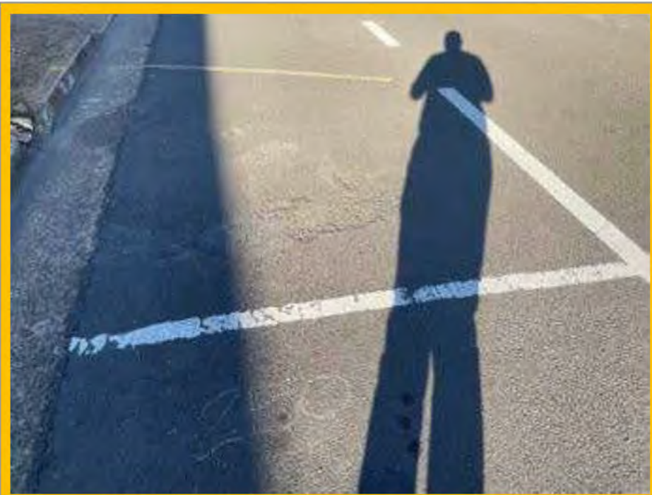
No. 044: depression in surface at approx. 251m
