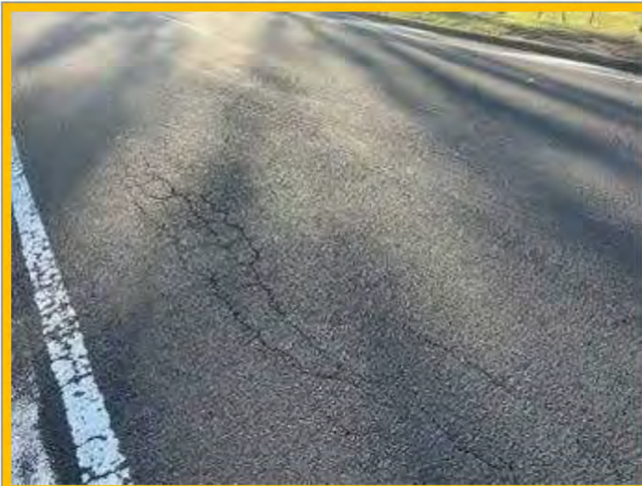
No. 045: cracking and deterioration of road surface from 210m to approx. 217m
