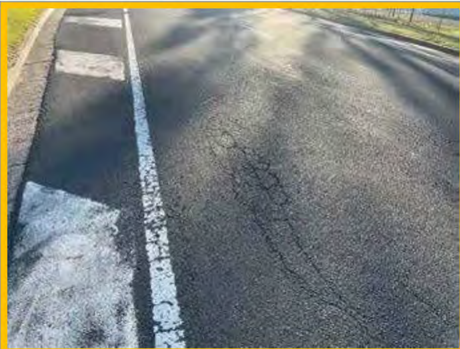
No. 046: cracking and deterioration of road surface from 210m to approx. 217m
