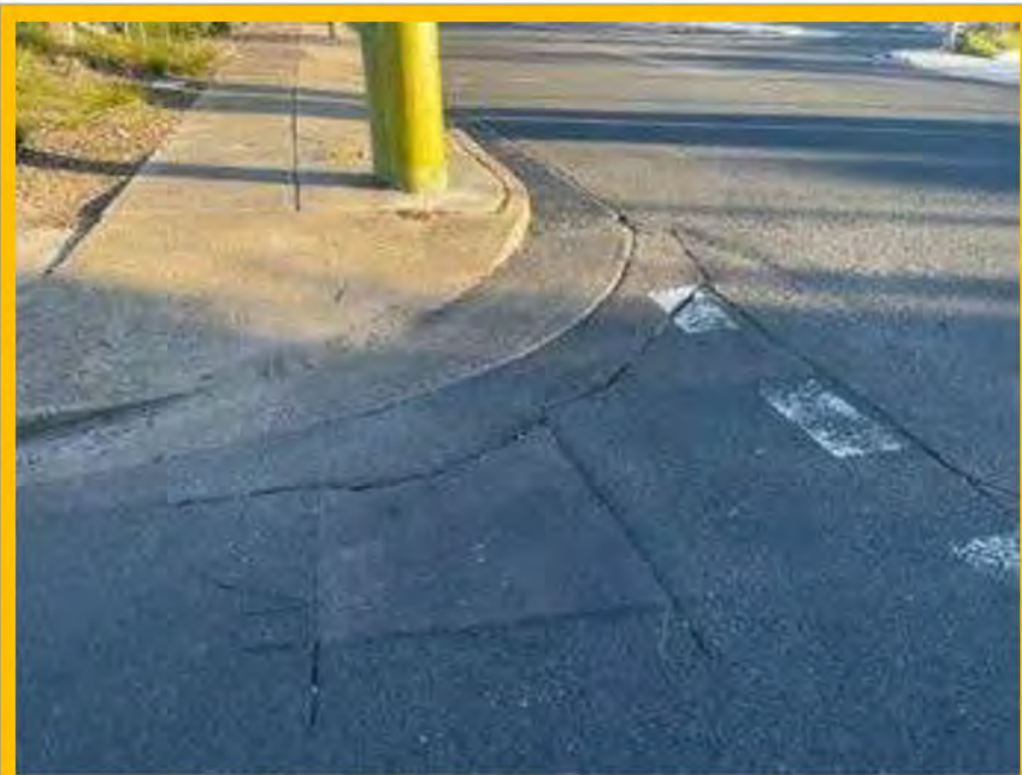
No. 129: depression and cracking to road surface at joints in road materials for previous repairs
